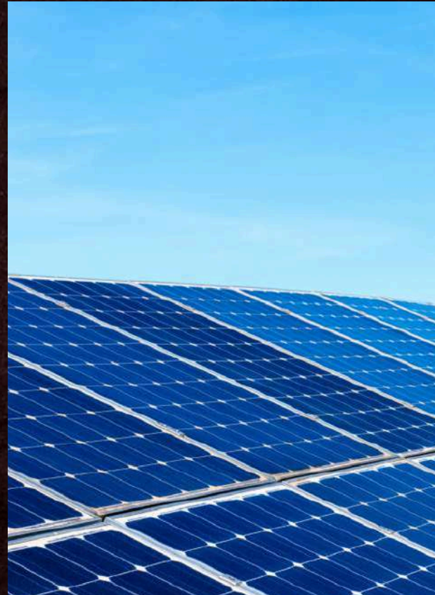
Solar Panels for Energy
